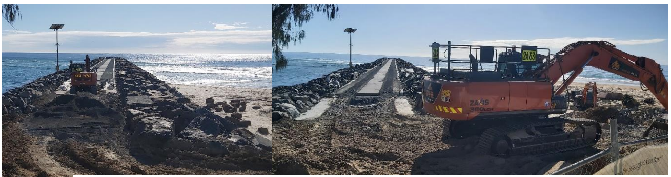
This year saw significant works to widen and stabilise the rock wall in the creek mouth.
